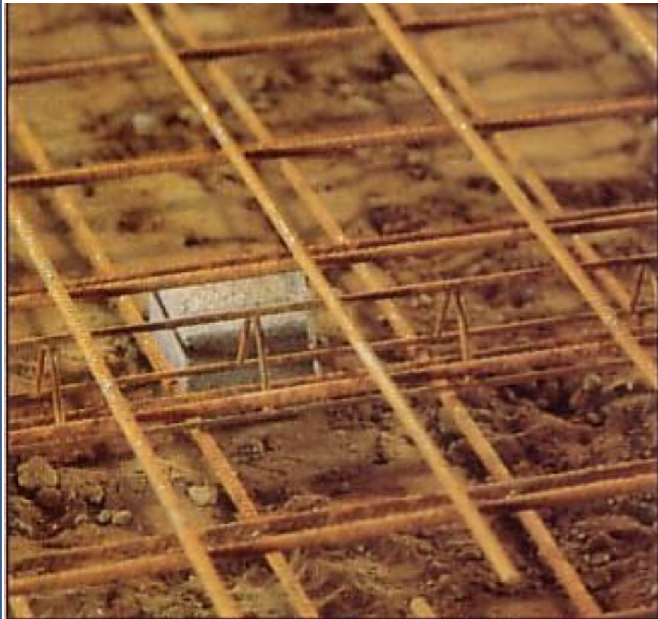
Concrete block (used to support bottom layer) Wire chairs (used to support top layer)
